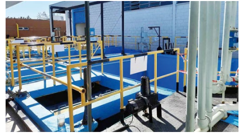
Wastewater diagnosis setup
