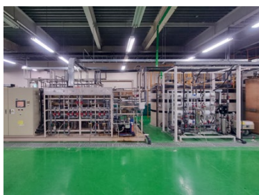
Water recycling at an overseas plant
