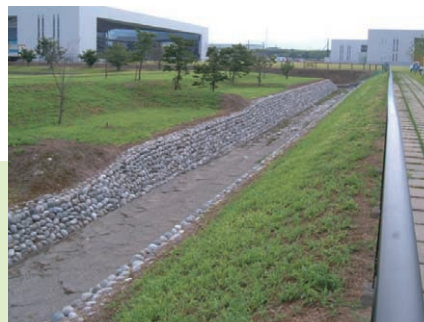
Rainwater permeable gutter
