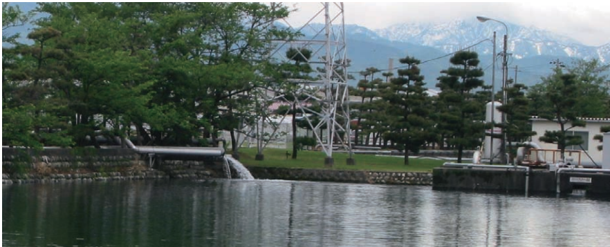
Cooling water collection pond with permeable stonework boundaries
