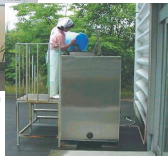
Reduction-type garbage disposal unit for disposing of garbage from the company cafeteria
