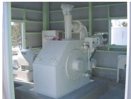
Tohoku Plants hydroelectric equipment using industrial water
