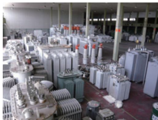
Storage for equipment containing low concentrations of PCBs, Kurobe office
