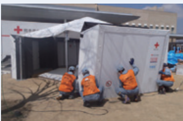
YKK AP Employees erecting a QS72 unit for use as a medical treatment room on the grounds of Ishinomaki Red Cross Hospital
