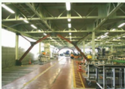
Reinforcement construction for earthquake resistance at the YKK AP Shikoku Plant Building
