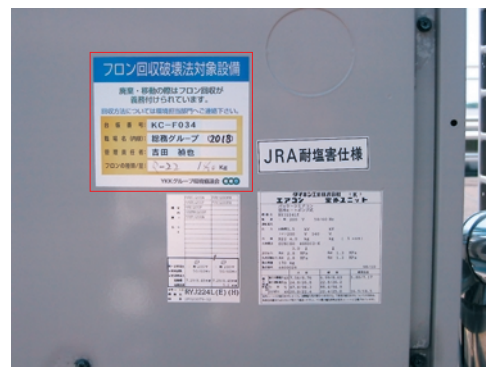
Management sticker applied to outdoor air conditioner unit
