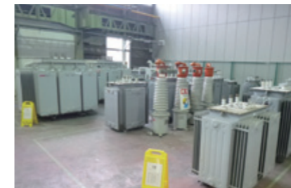
Storage of equipment containing low PCB concentrations (Kurobe Manufacturing Center)
