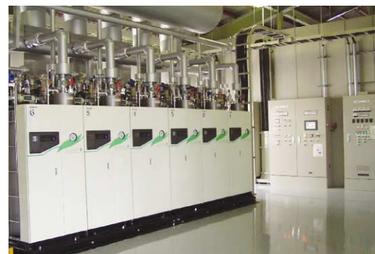
Small high-efficiency LPG-burning once-through boilers (6)
