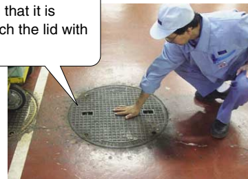
Indoor hot water tank (underground)
