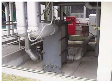
Pre-existing outdoor heat exchanger
