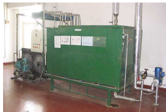
Circulatory cooling equipment
