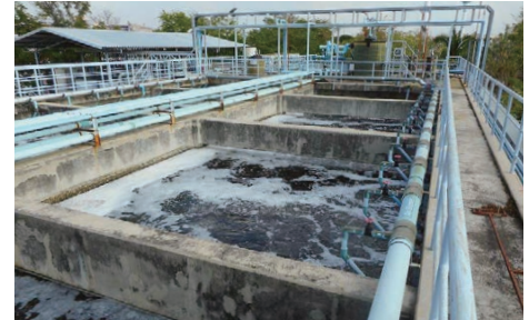
Wastewater processing and diagnosis setup at YKK (Thailand) Co., Ltd.
