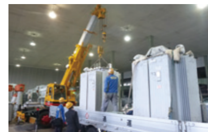
The removal of equipment containing low concentrations of PCBs at the Kurobe Manufacturing Center
