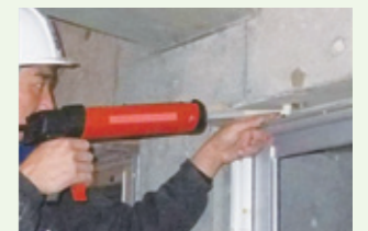
Sash installation using high-strength resin (Injecting resin adhesive to fix a sash)
