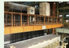
Combustion chamber's heat retention improvement
