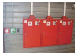
Fire and smoke control system
