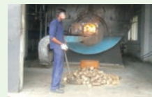
Biomass boiler (India)
