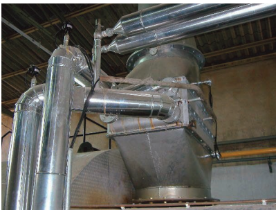
The water supply for the boiler is preheated using the heat emitted from the boiler (YKK España)
