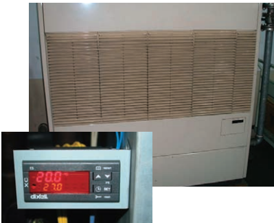
Temperature control equipment has been added to all 179 air-conditioners in this factory (YKK Taiwan)
