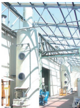
We installed two purification equipment units that neutralize hydrogen cyanide gas using sodium oxide solution (YKK Mediterraneo)
