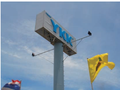
Outdoor lights have been replaced with energy conserving types (YKK Thailand)
