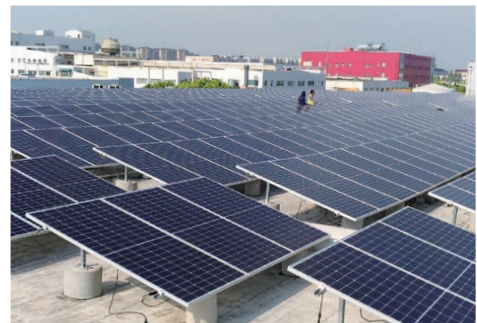
Solar power generation at Shanghai YKK Zipper
