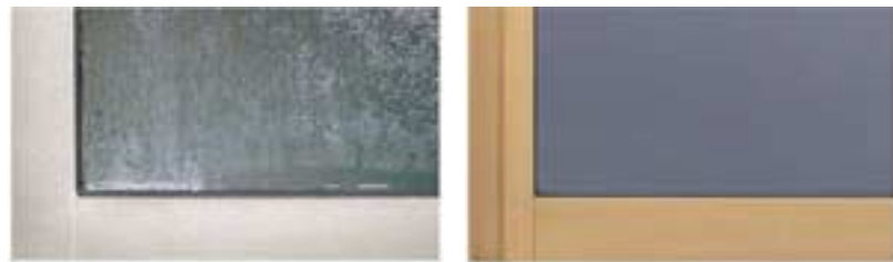
Aluminum window frame (Freming II) + single pane glass Aluminum and resin window frame (Apsword) + Low-E double pane glass Condensation on glass and sash with water droplets running down window No condensation on glass or sash
