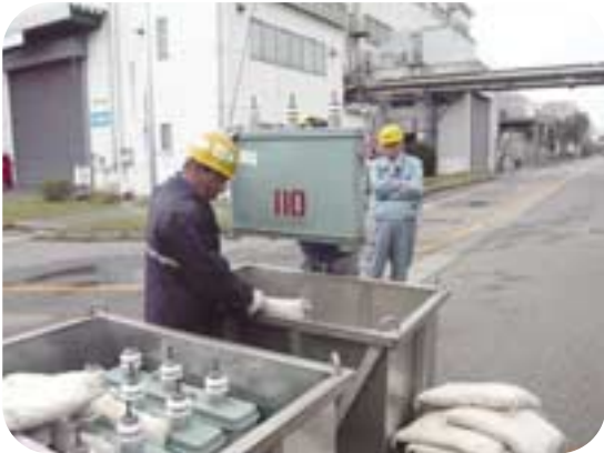
Moving equipment containing high-concentration PCBs
