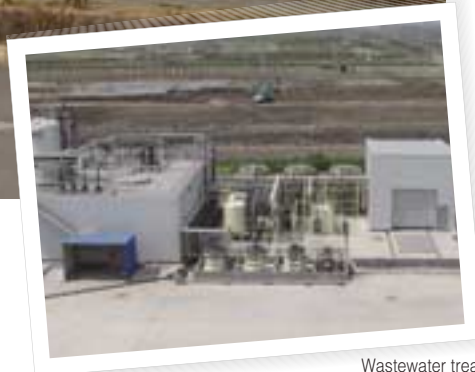
Wastewater treatment and recycling equipment
